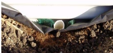
Photo 8, drain pipe. trickling out.
